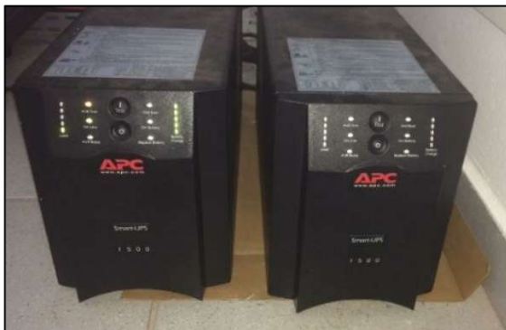
Nobreaks - Rack. - 24 H Alberto Kallas
