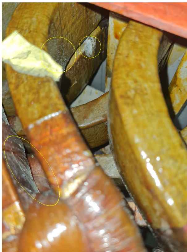
Figure 80 – Corona spots prior to repair, slot 37.
