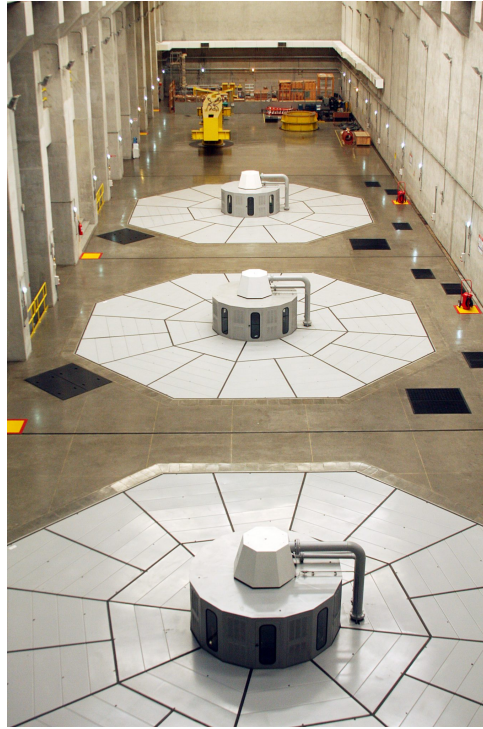
Figure 19 – Power house of the Enercan hydro plant.
